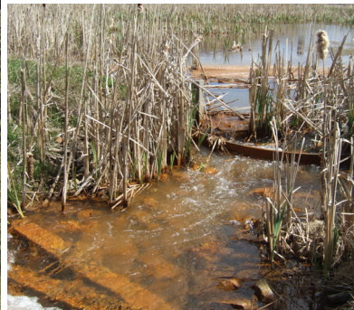
Treated clean water exits the final wetland filtering pond and enters Sewickley Creek.
