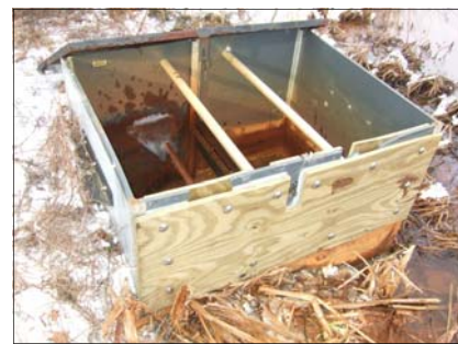
This damaged water level control structure was repaired, thanks to Michael Pacacha's Eagle Scout Project at the Brinkerton remediation site.
