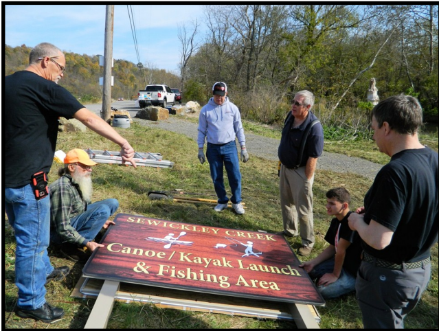
Volunteers from Firestone Building Products, Westmoreland Conservation District, Yough High School and SCWA work together to install the new Lowber Canoe/Kayak Access sign.
