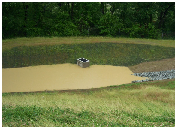
Three retention basins were created to control runoff and sediment from the Fairgrounds arena, parking and road areas.
