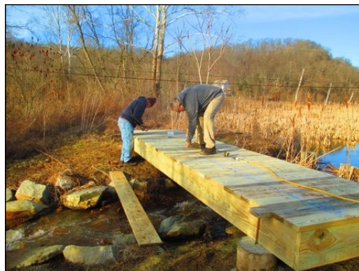
Board members Ted Curnow (front) and Darl Dodson install decking on the bridge.
